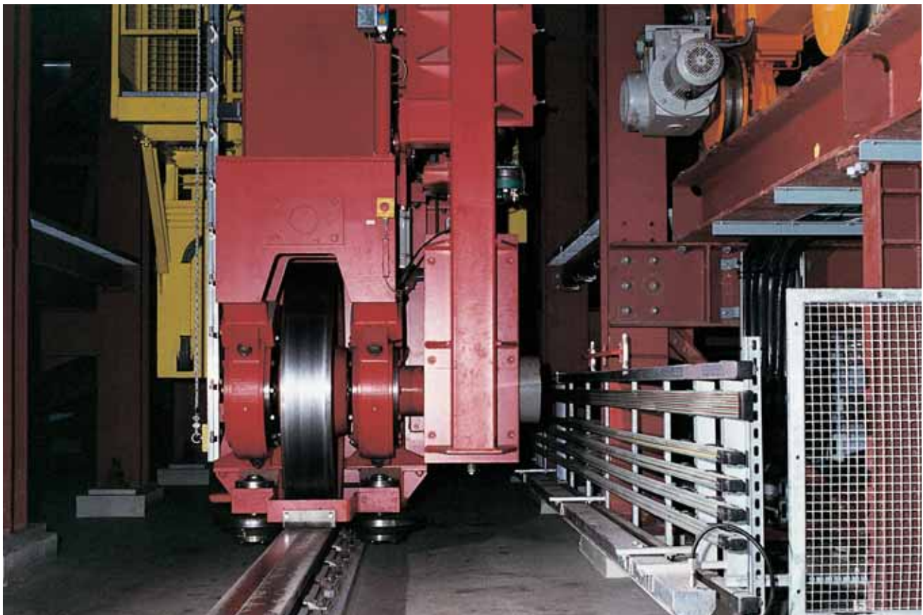
SMG-Data Transmission with VAHLE Conductor System for AS/AR warehouse
